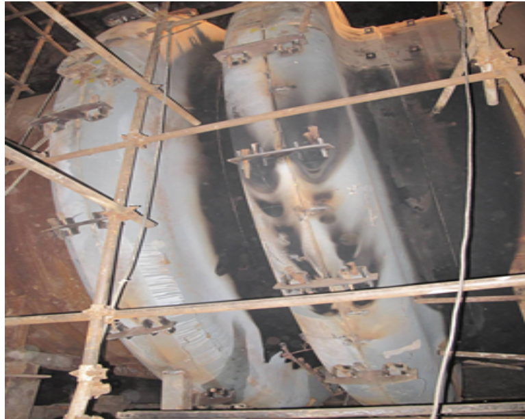
Figure 7. implemented steel lining in the Siah Bisheh project with a special design at the creativity stage of value engineering studies (17)
