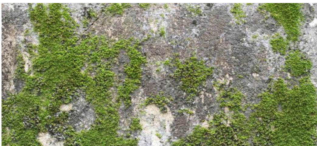
Figure 1. The proliferation of marine organisms on concrete components
