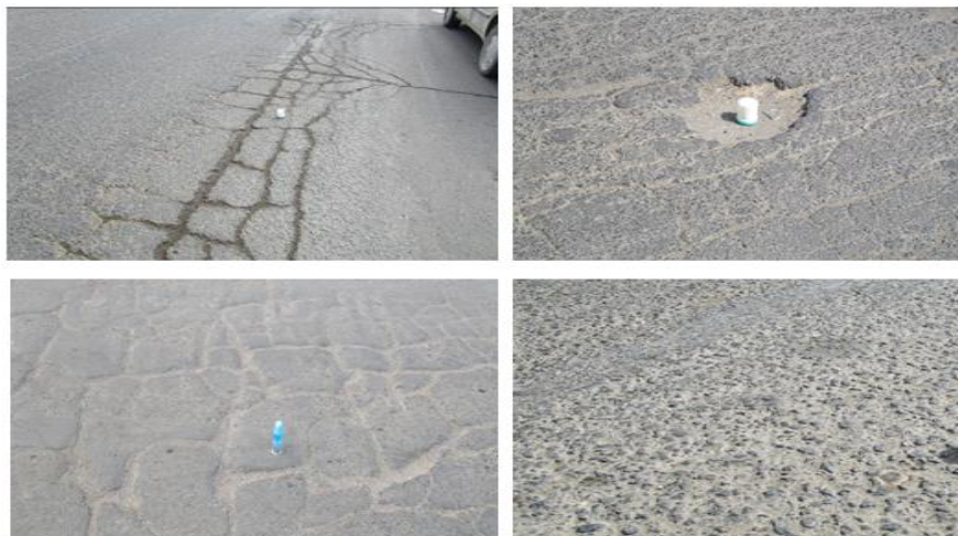
Figure 1. Some of the pavement failures on Sirjan streets.
