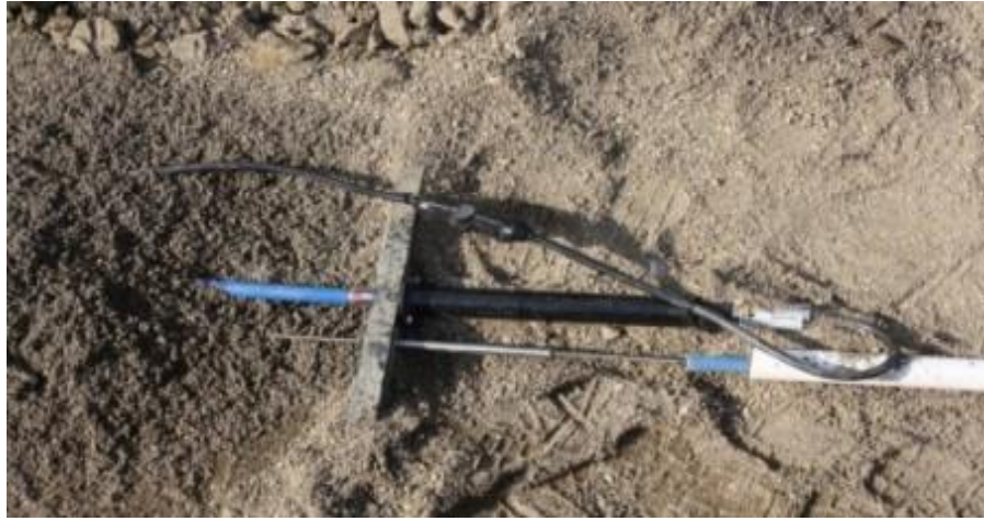
Figure 16. Channel connected to sensor of extensometer in Shahr-e-Bijar Dam
